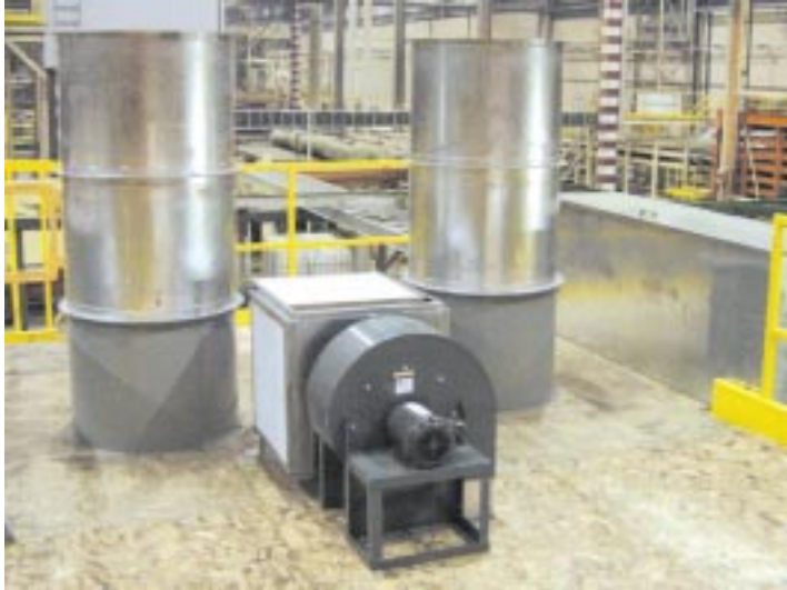
Top of booth has space for fans, ducts and filter storage.
